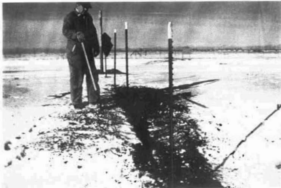
Figure 4. Installation of posts for a snow fence on Block 1 of the BP Put River No. 1 gravel pad experimental area (25 September 1990).
