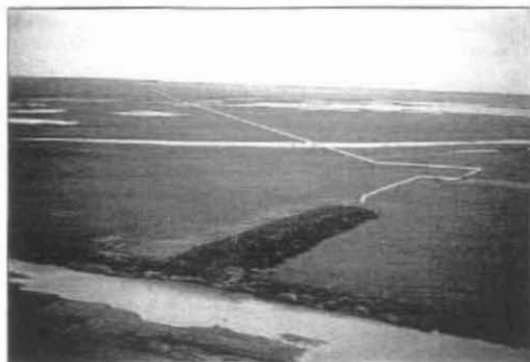
Figure 4. Low angle aerial oblique view westward of west end of Badami Pipeline crossing of the Kadleroshilik River (27 August 1999). Peat and silt overburden used to cap the backfilled trench for the buried section of the pipeline appears dark, in contrast to the light-colored gravel fill around the riser pipe and for the helipad and check valve. Vegetation is moist rhizomatous sedge/Dryas meadow. In the distance, an old river terrace is apparent. Gravel fill at this location was seeded and fertilized 31 July 1999 (McKendrick, 2000).
