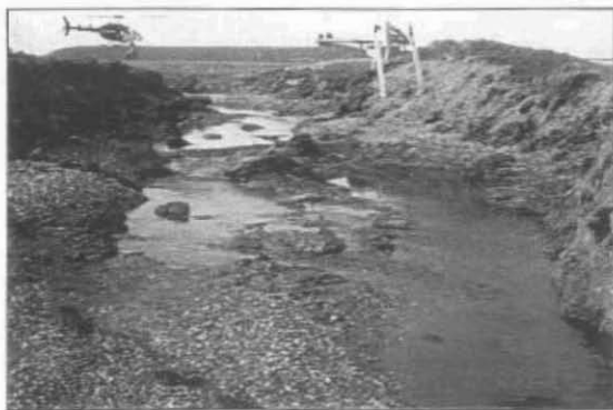
Figure 11. View westward up the gully cut through the backfill over the buried pipeline at the west end of the Sagavanirktok crossing for the Badami Pipeline (27 August 1999).
