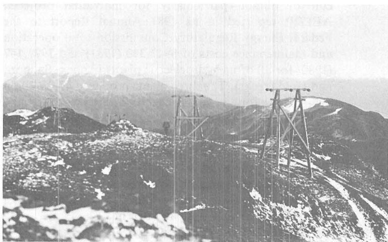
Figure 19. The Annex Creek transmission line near Juneau was often subject to outages due to the mountainous, avalanche-prone terrain it traversed. The line first supplied power in 1915. These photographs were taken in 1940.
