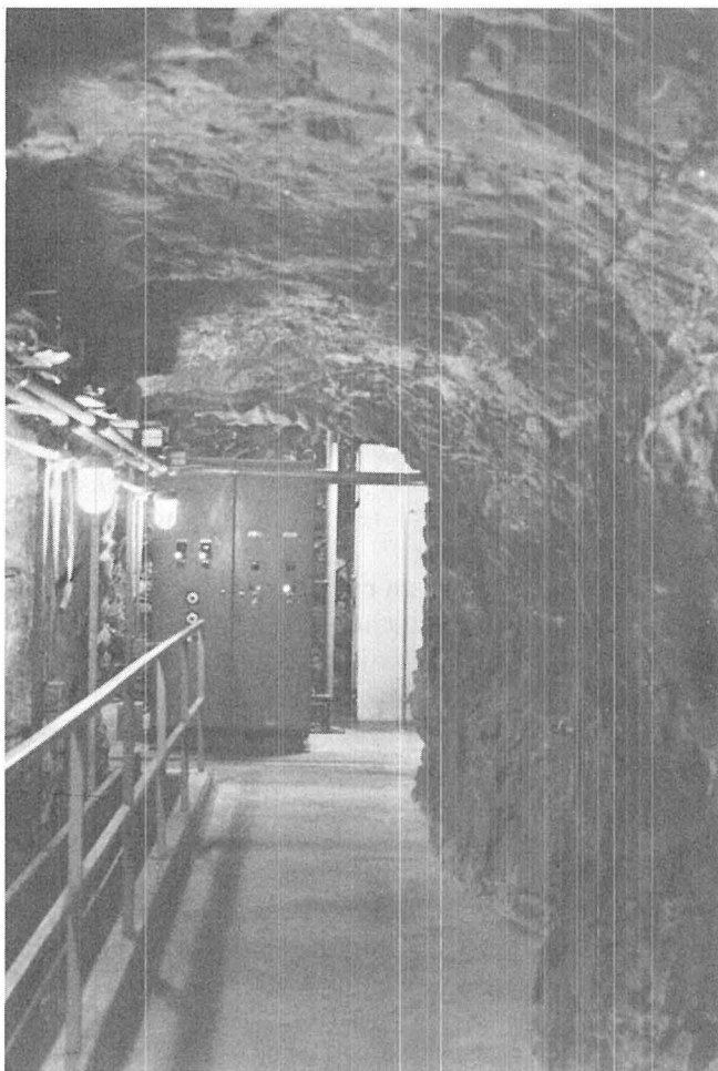
Figure 35. The Snettisham hydroelectric project near Juneau is noted for its underground powerhouse.
