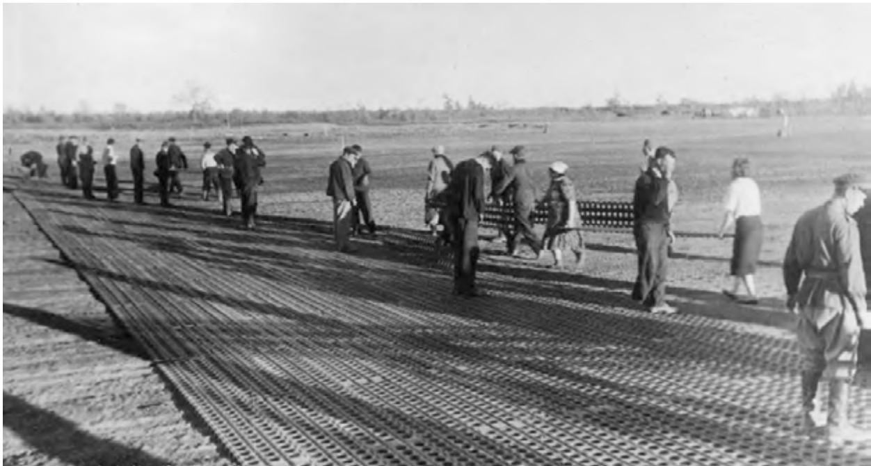
The laying of a metal runway at Tanyurer in 1944. Courtesy of Ivan Negenblya.
