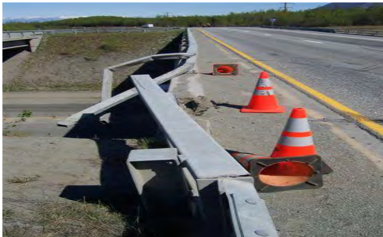
Figure 13. Bridge Railing Damaged by a Vehicle Collision
