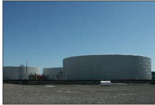
Water storage tanks
