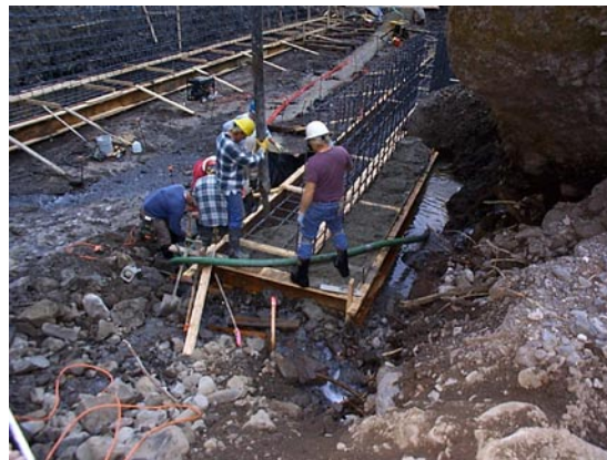
Fig. 6. Concrete is being placed to seal off water at upstream end of form first.
