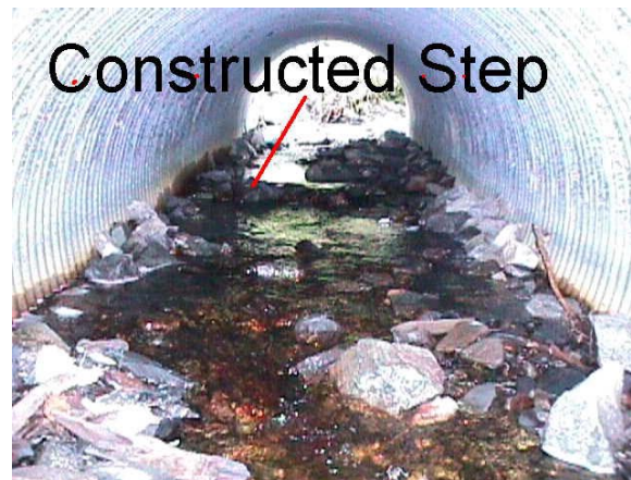
Fig. 8. Constructed step and boulder groups at margins inside culvert similar to Demo Cr.
