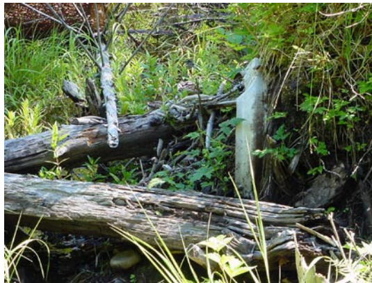
Fig. 3. Woody debris plugging culvert inlet.
