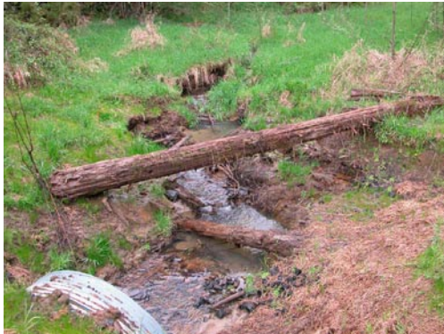
Fig. 15. Administration Problem - Survey error leads to wrong inlet elevation.
