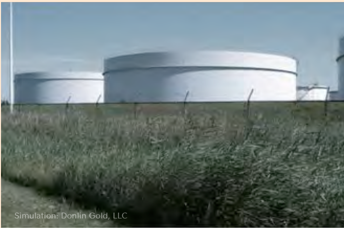
Typical Fuel Storage
