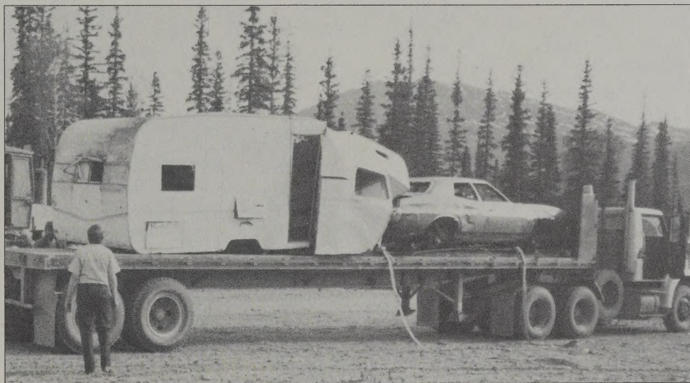
Workers from the Alaska Department of Transportation hauled away big items like vehicles, trailers and tractor tires, using equipment loaned by the Alyeska Pipeline Service Company.
