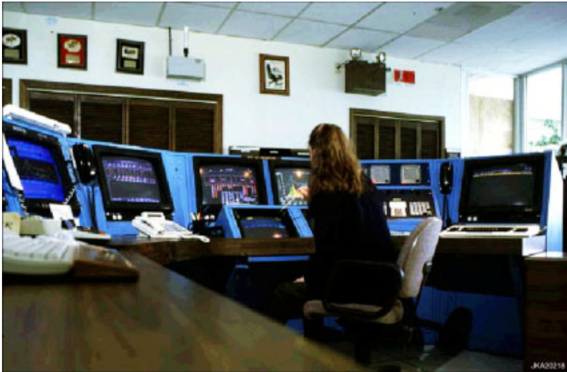
FIGURE 3.1-2 Operations Control Center at Valdez Marine Terminal (Source: TAPS Owners 2001a, Photo 2.1-3)
