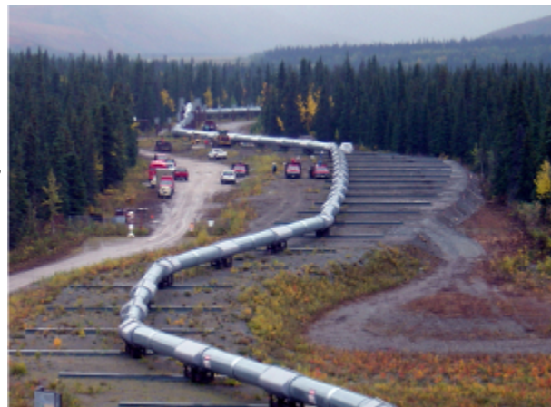
The trans-Alaska oil pipeline, where it crosses the Denali Fault, is designed to move 20 feet laterally and 5 feet vertically. Source: Alyeska Pipeline Service Co.
