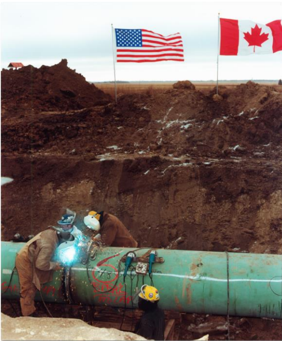
On Nov 30, 1999, workers welded the Alliance Pipeline where it crosses U.S.-Canada border. Photo courtesy of Alliance Pipeline.
