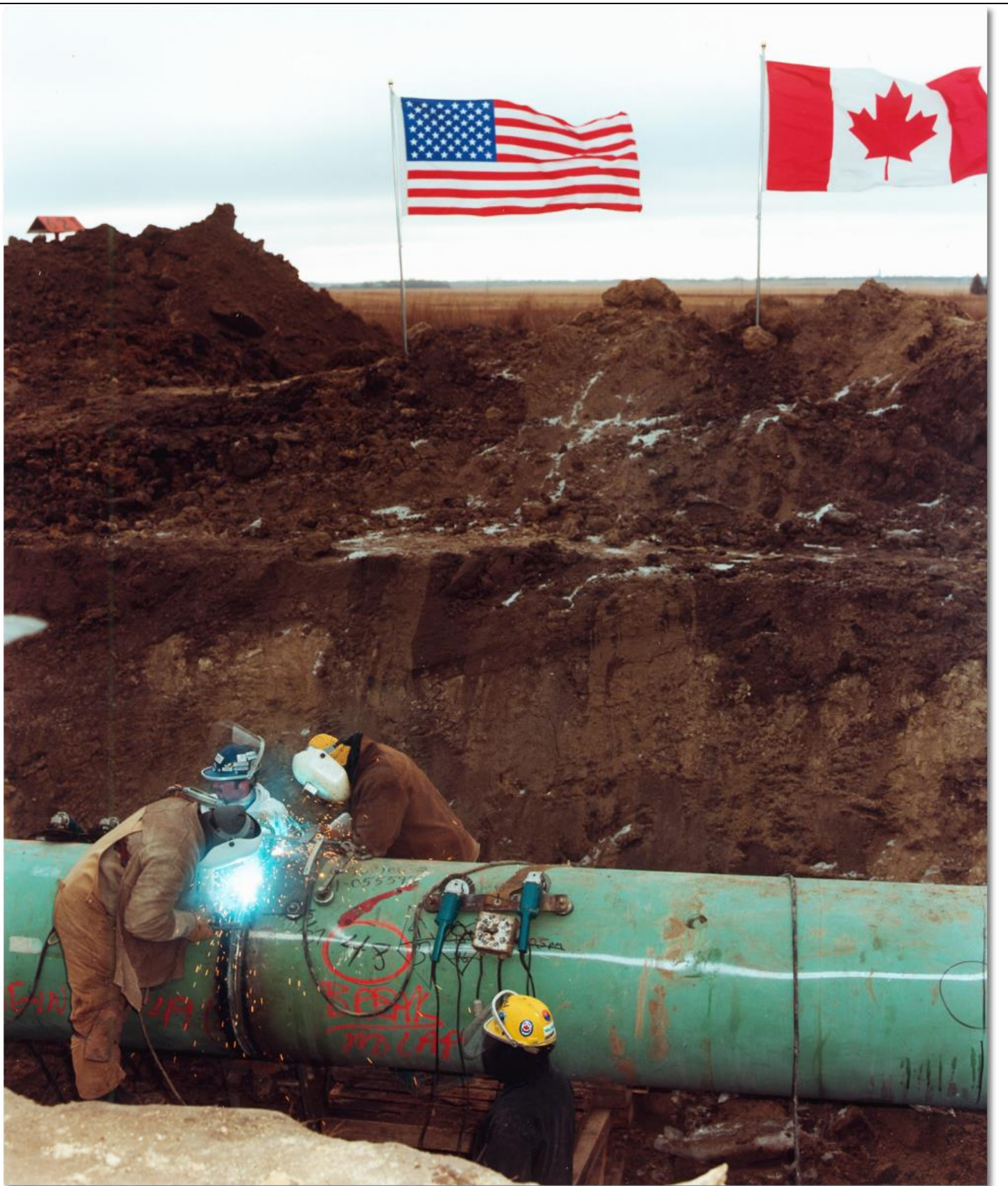
On Nov 30, 1999, workers welded the Alliance Pipeline where it crosses U.S.-Canada border. Photo courtesy of Alliance Pipeline.
