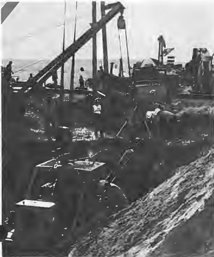
Pipe is installed across a railroad near Piapot, Saskatchewan using a "slip bore." Powered by the machine in the foreground, an auger inside a length of pipe bores a tunnel under the railroad. The pipe is then pulled or "slipped" out and the "carrier" or permanent piece of pipe is put in.
