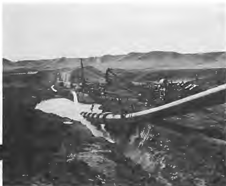
Sideboom tractors lower the pipe into the trench in the bed of the Frenchman River in southwestern Saskatchewan.
