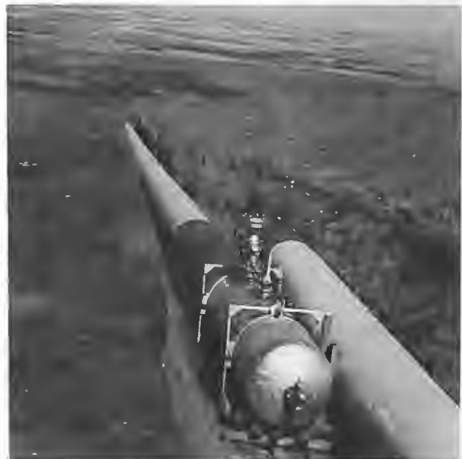
A completed pipeline section is ready for hydrostatic testing near Piapot, Saskatchewan. Heavy-walled test heads welded onto the pipe end are designed for safety as the water inside the pipe is pumped to test pressure — a minimum of 10,863 kilopascals (1,575 lb. per sq.in.).
