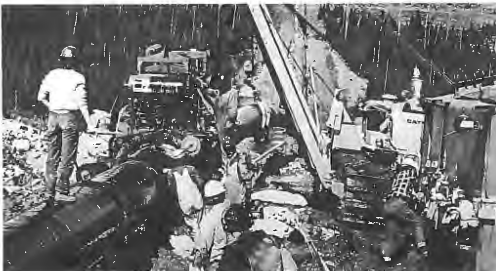
Construction of the Alaska Highway pipeline in South B.C. Photo by: Lee Burkitt (Daily Townsman)
