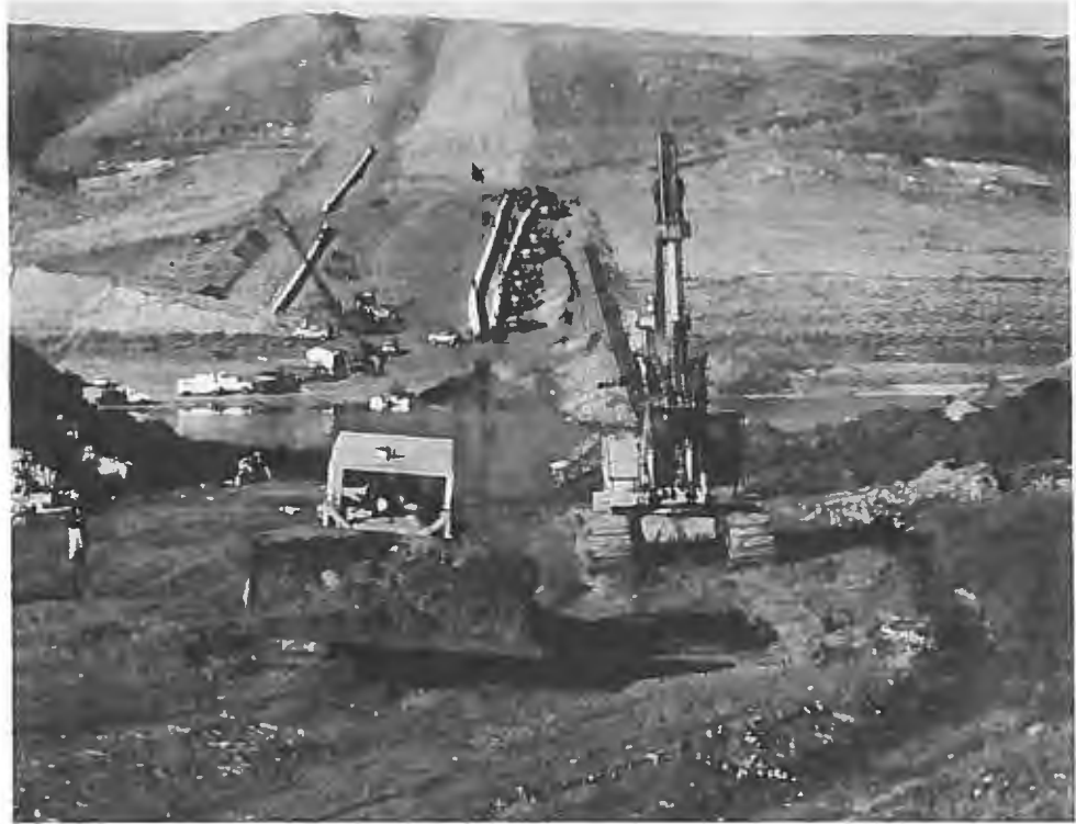
As sideboom tractors lower the first section of pipe into the water, a bulldozer anchored on the opposite shore pulls the pipe with cables.
