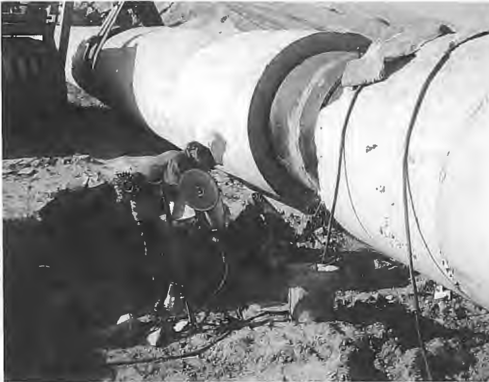
The two river sections of pipe are welded together on the west bank before the final pull.
