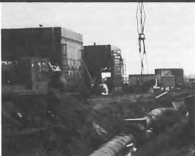
Installation of high pressure discharge piping at compressor station on Eastern Leg near Jenner, Alberta.
