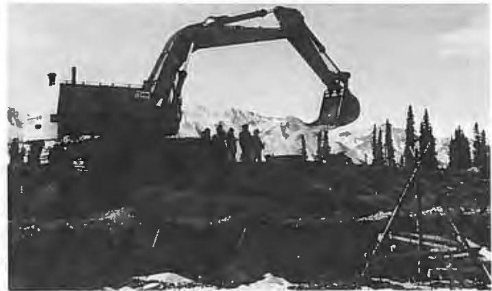
Backhoe covers pipe in embankment with gravel at Quill Creek test site.
