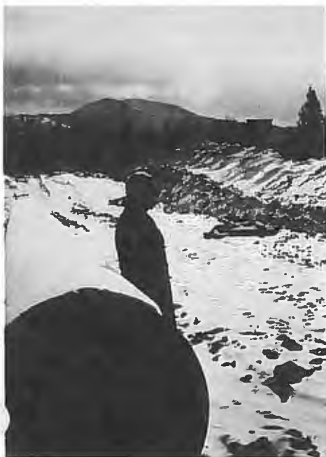
The Hon. Mitchell Sharp, Commissioner of the Northern Pipeline Agency, views U.S. Western Leg construction near Sandpoint, Idaho.
