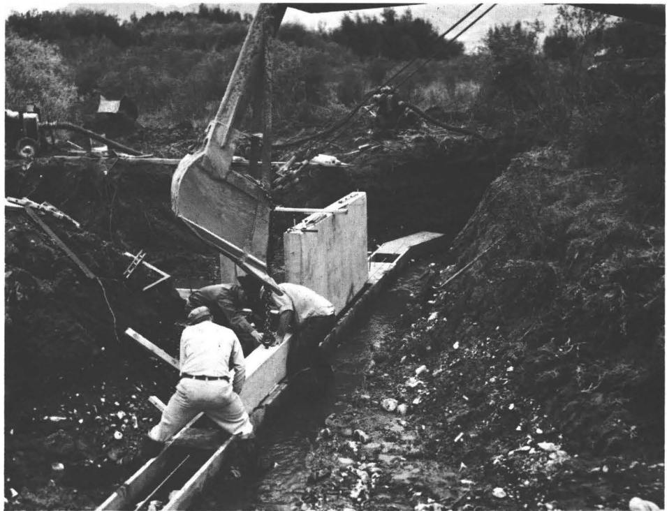
Figure 18.—Installing prefabricated wall sections of a vertical perforated-plate fish screen in the Pahsimeroi River drainage near Salmon, Idaho.
