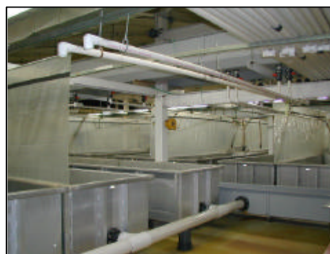
Main Bay Hatchery interior.
