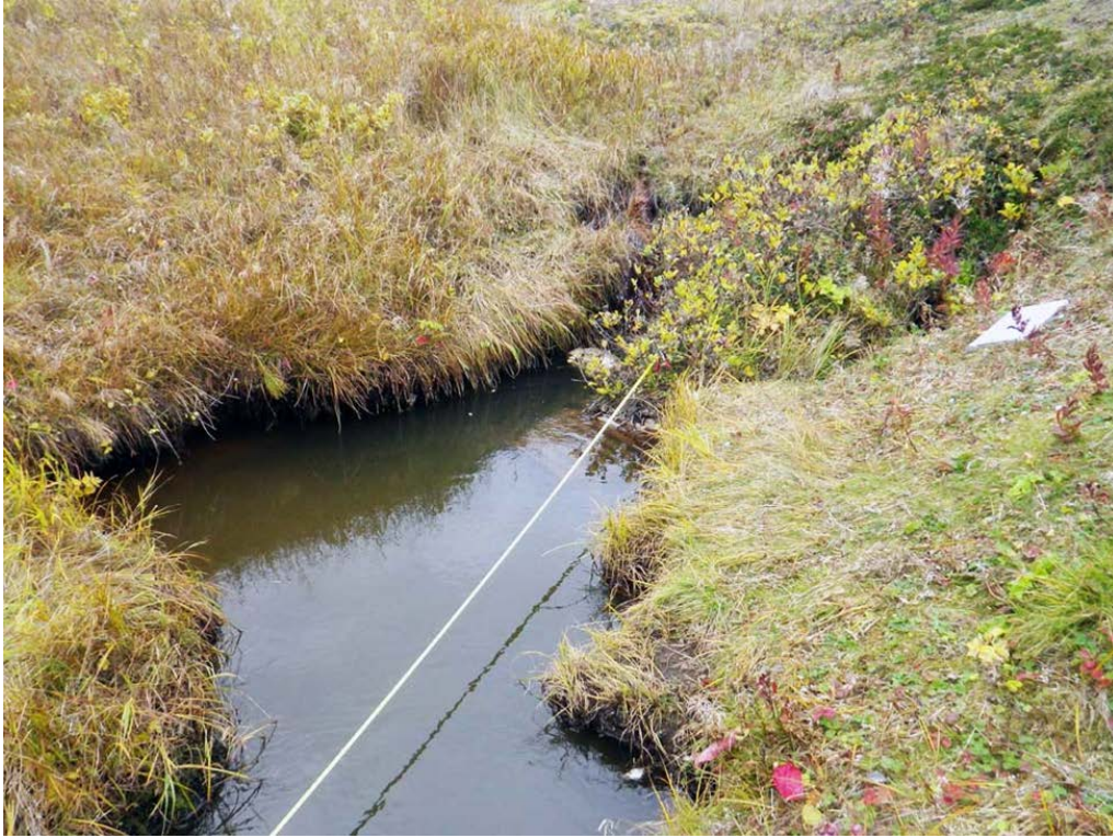
Figure 10.—Site 30103341, unnamed tributary to Trout Creek on the airport runway light access road, damaged inlet.
