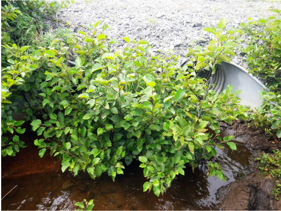
Figure 41.—Site 30103460, culvert inlets, C1 (left hand side) taking almost all flow.
