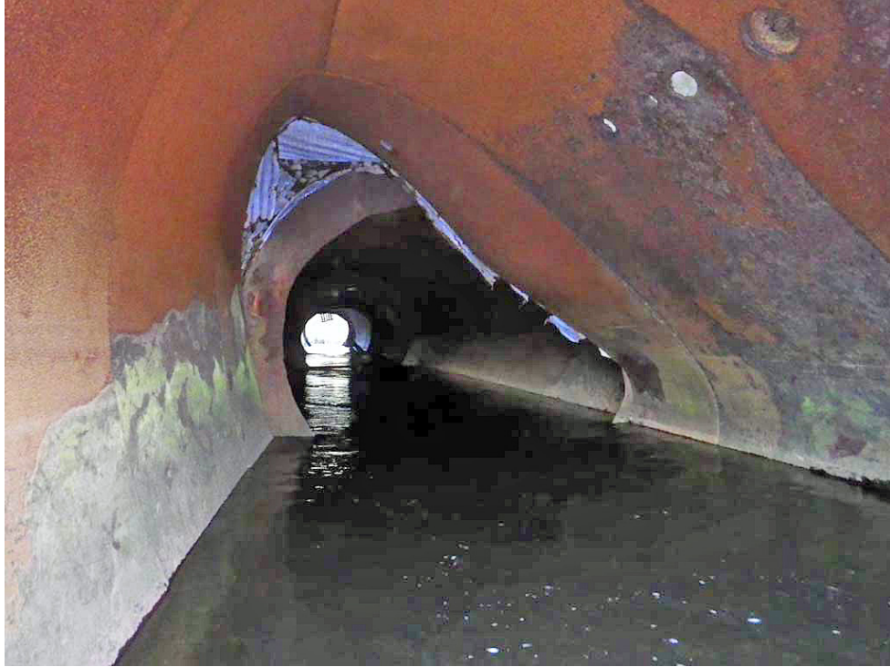
Figure 17.—Site 30103336 inside culvert looking upstream from outlet showing internal structural problems and internal baffles from tank lips.
