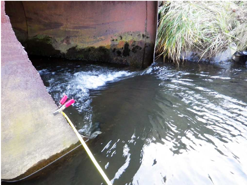
Figure 16.—Site 30103336, stream constriction at inlet creating a hydraulic jump, inlet.
