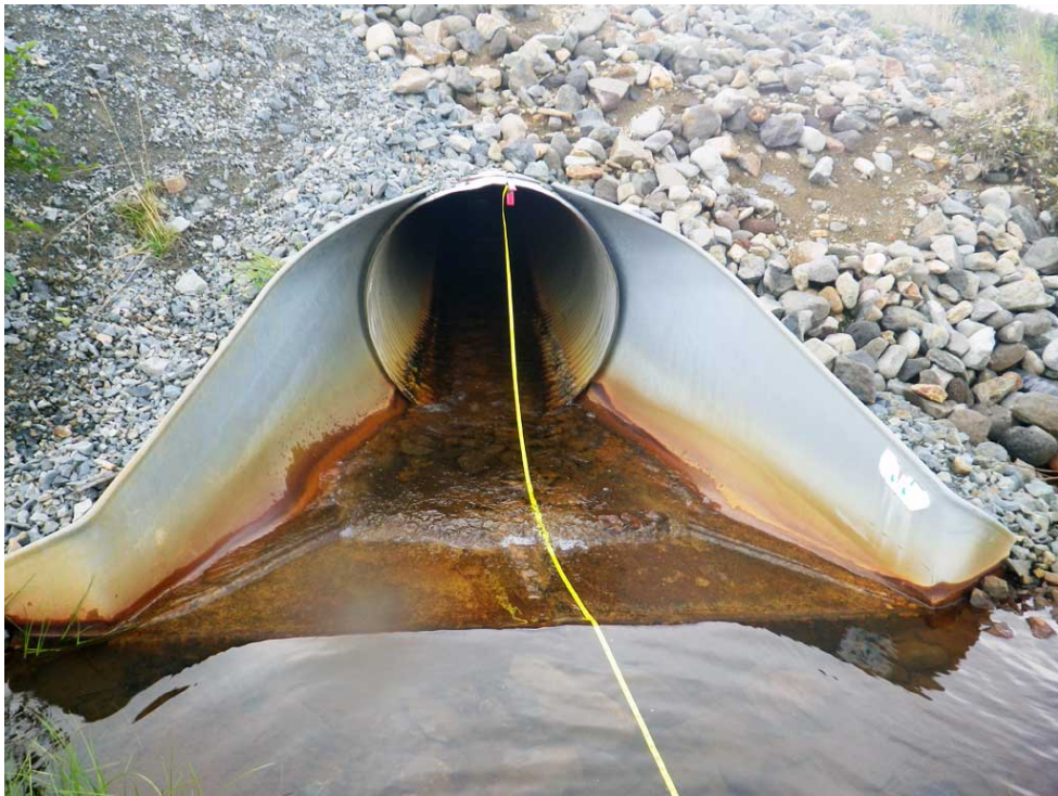
Figure 45.–Site 30103459, culvert inlet, showing inlet perch.
