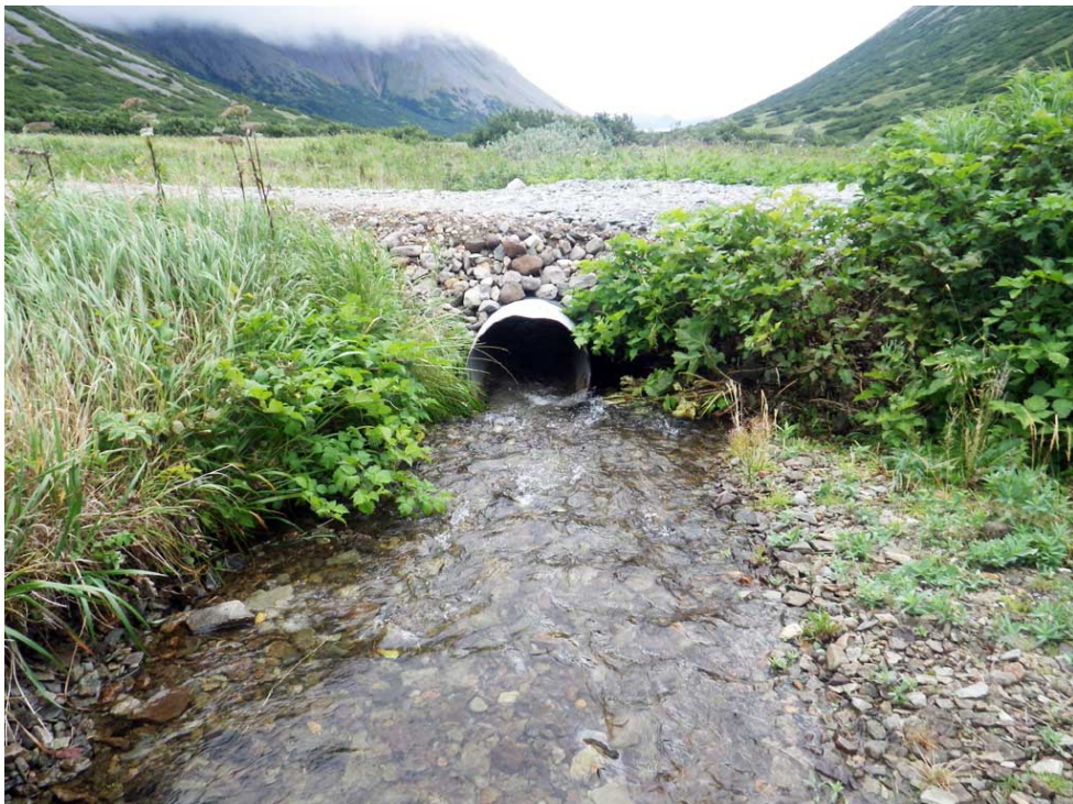
Figure 36.—Site 30103448, constricted culvert inlet.
