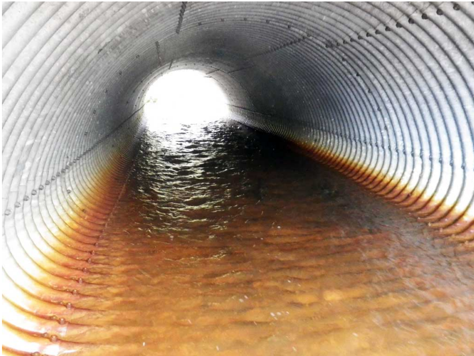
Figure 31.—Site 30103446, interior of culvert showing water level and rust line.
