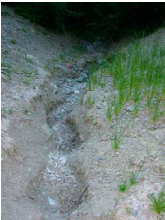
Photo 1: Typical stream crossing erosion due to post-treatment channel incisement.
