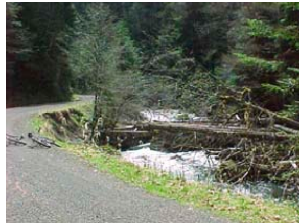
Figure 5: The Upper Dungeness River at the 2860 Road washout. Boulders in mid-channel and the constriction formed by the road encourage accumulation of logs and diversion of flow along the toe of the fill. This has been a chronic problem area.
