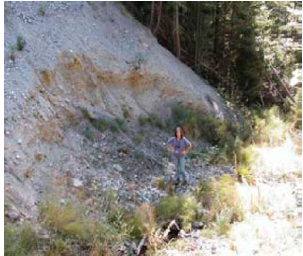
Photo 4: Channel bank failure due to oversteepened slope and inadequate channel width.
