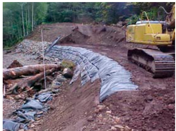
Figure 7: Construction at Walter Creek. Note the installation of geotextile fabric reinforcement through steepened section of the revetment.
