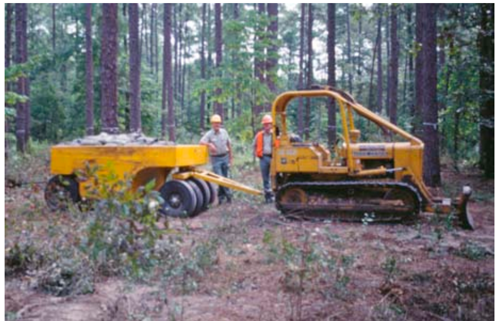
Figure 3. Wobble-wheel road compactor and dozer used to compact soils in the western Gulf Coastal Plain Long-Term Soil Productivity sites. Photo by Allan Tiarks.
