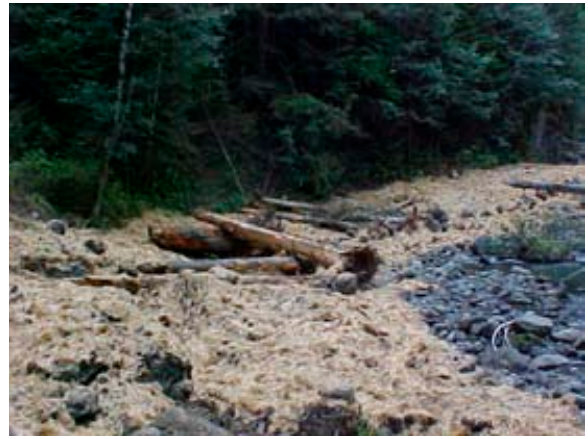
Figure 6: High intensity decommissioned section through former washout; roadway and all associated fill have been removed. Straw mulch indicates former road and area disturbed by excavation. Two of the log complexes placed for structure and stabilization can be seen on the left. Note the lower intensity of treatment at the far (upstream) end.
