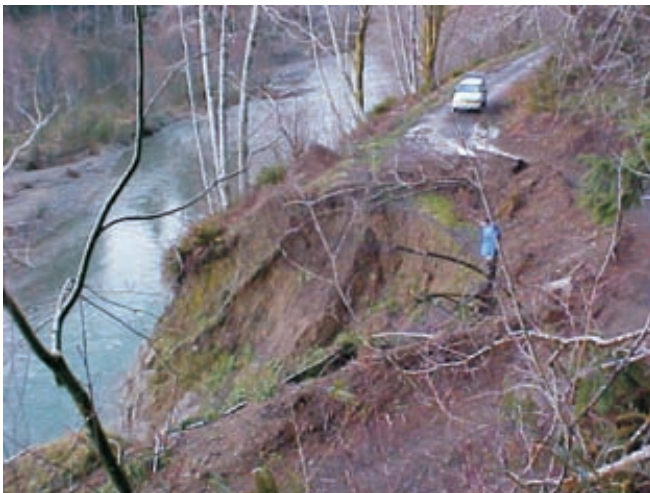
Figure 2. Encroachment within an active landscape: North Fork of Calawah River, Forest Road 2923. Assessment included evolving or active slope processes at washout.
