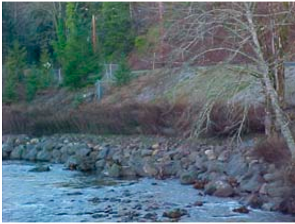
Figure 9: Big Quilcene River revetment just upstream of Highway 101. Note the irregular shaped rock toe incorporating rootwads and built to a limited height with brush layers installed above.
