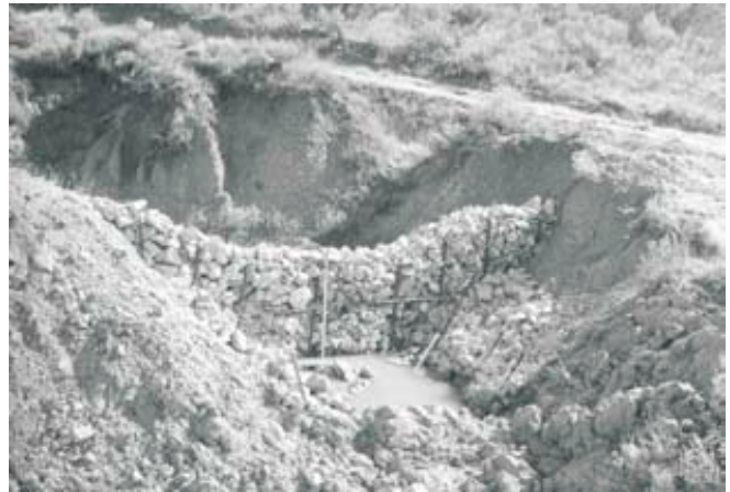
Figure 9. Typical double fence check dam. Photo by B. Heede.
