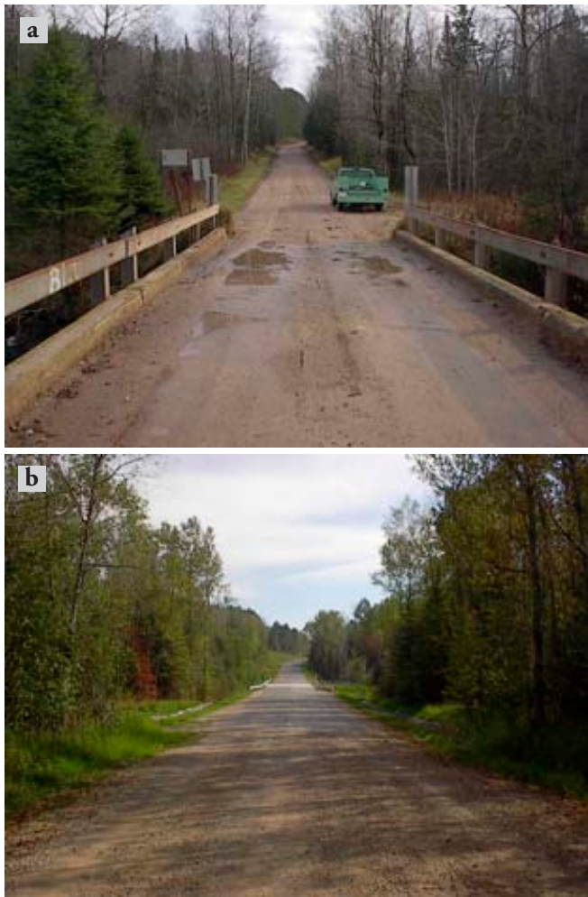
Figure 3. Sturgeon River Bridge, Hiawatha National Forest, Upper Peninsula of Michigan. (a) Before, (b) After. Former road was narrow, with native road surfacing material; stream crossing was at the lowest elevation on the road and this allowed runoff to flow down the road and deposit sediment into the Sturgeon River, a cold-water, low gradient stream. The new crossing was slightly elevated, provided more sunlight to the roadbed; the bridge was replaced; the approaches and crossing were hardened and runoff drains were constructed. Photos by Richard Kell.
