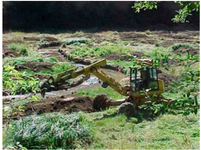
Figure 7. Channel construction in lower Karnowsky Creek with a walking backhoe, summer 2002. Fill material taken from the constructed channel was shaped into floodplain hummocks that would later be planted with native trees and shrubs.
