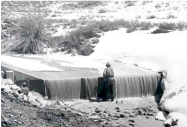
Figure 12. (a) Precast concrete check dam at the base of the main gully during spring runoff in 1964. Photo by B. Heede. (b) The same structure during the early summer of 2004. Photo by C. Hirsch. Note that the right half of the structure is covered by willows.
