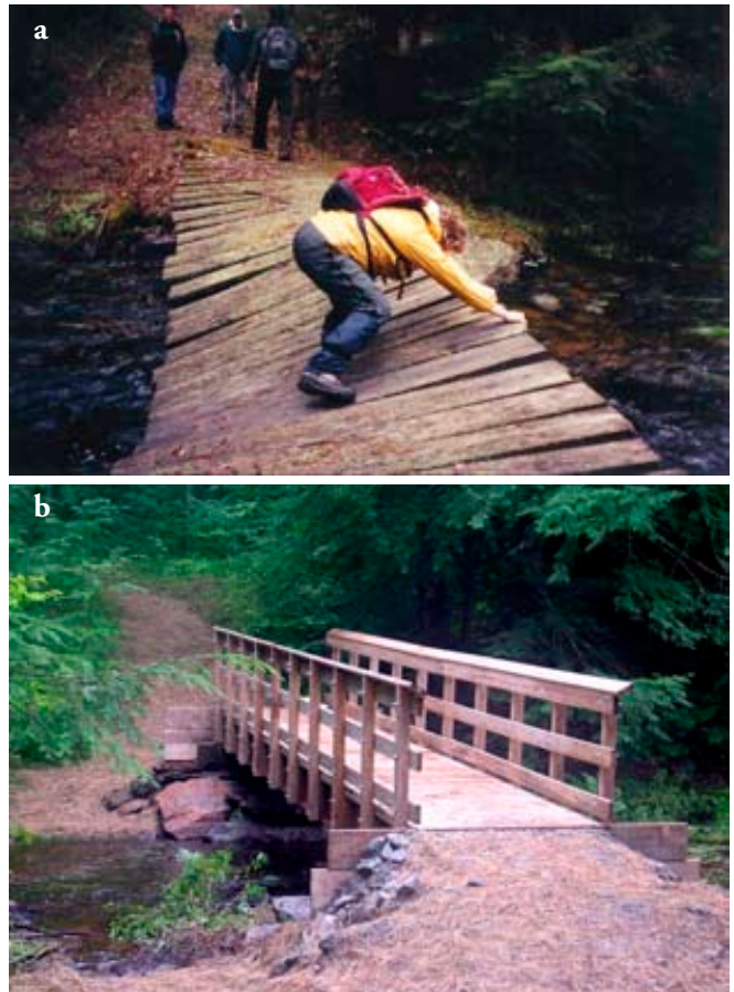
Figure 4. Burnt Meadow Brook Bridge replacement, Catamount Trail, Green Mountain National Forest, Vermont. (a) Before, (b) After. Photos by Richard Gaiotti.
