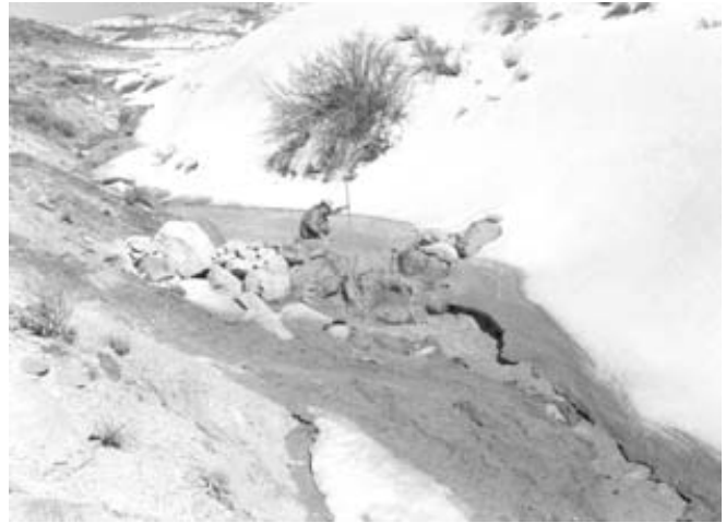
Figure 13. (a) Rock check dam on the main gully (structure M5) during spring runoff of 1964. Photo by B. Heede. (b) Same rock check dam in the fall of 2004. Photo by M. Weinhold.
