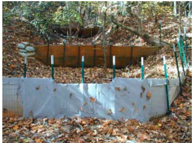
Figure 8. Additional dams were added to capture sediment. After 4.5 years (February 1999), a total of 40 tonnes of sediment were captured for an average sediment yield of 89 tonne \text{ha}^{-1} \text{yr}^{-1} (36 tons \text{ac}^{-1} \text{yr}^{-1} ). Most of the sediment was delivered during three major tropical storm events.
