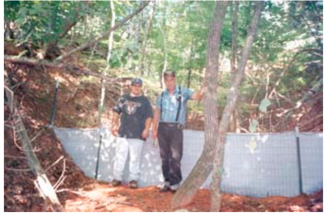
Figure 5. The fabric dam was installed in July 1994 below the 0.1-hectare ephemeral gully. The filter fabric was supported with steel posts, wire fencing and C clamps.
