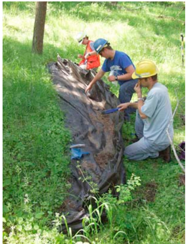
Figure 2. Example of a sediment fence. The fence is 5 meters wide, 0.5 m tall, with a 0.8 m long apron. The upslope edge of the apron is buried in a shallow trench. See Robichaud and Brown (2002) for installation details.
