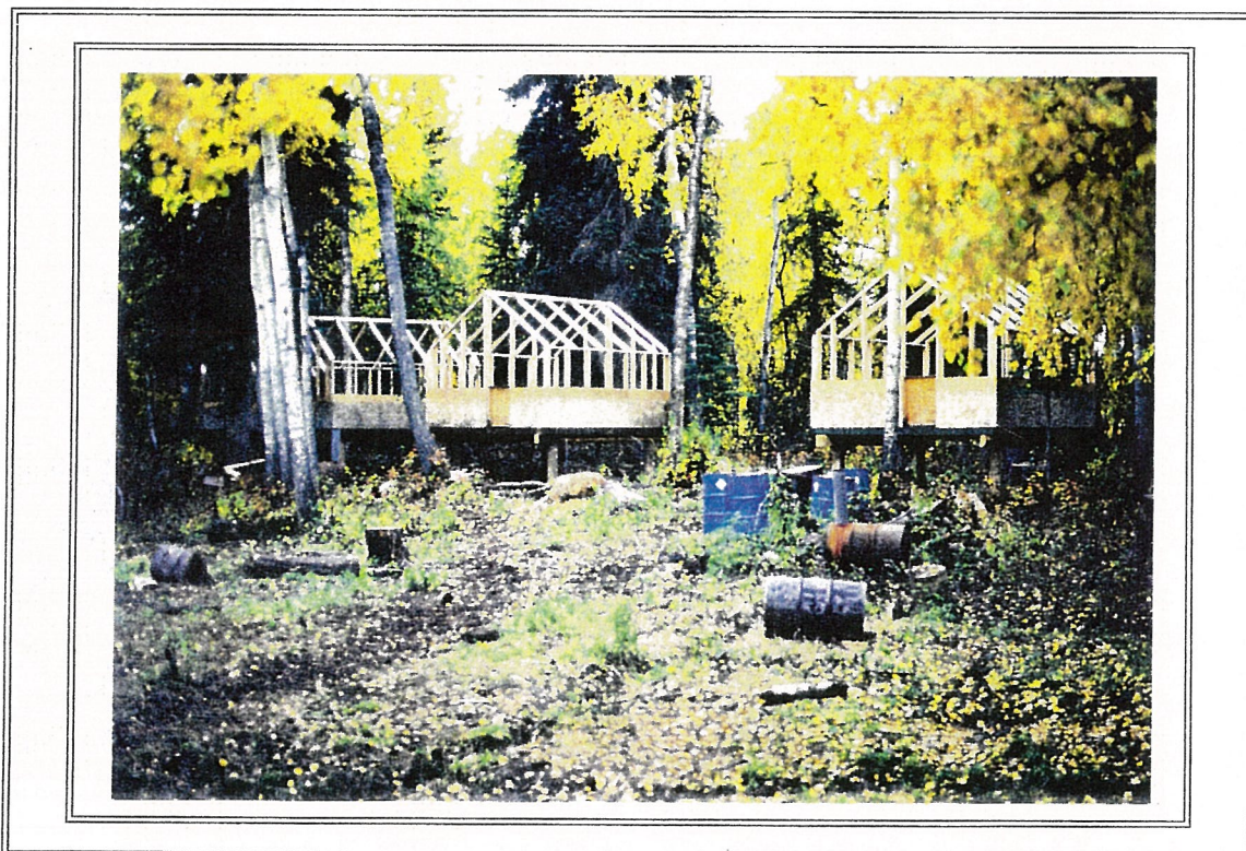
Raising these tent frames one foot above flood stage will alleviate the need to reposition them every spring (BA 9/94).
