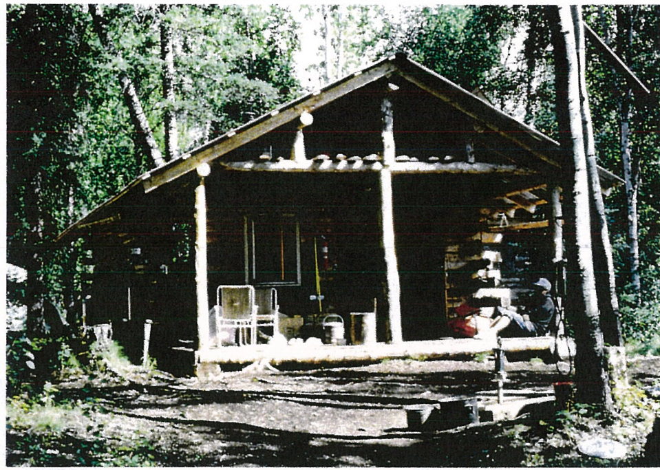
At this level the cabin was continuously flooded for several years causing damage to the structure and equipment (7/92).
