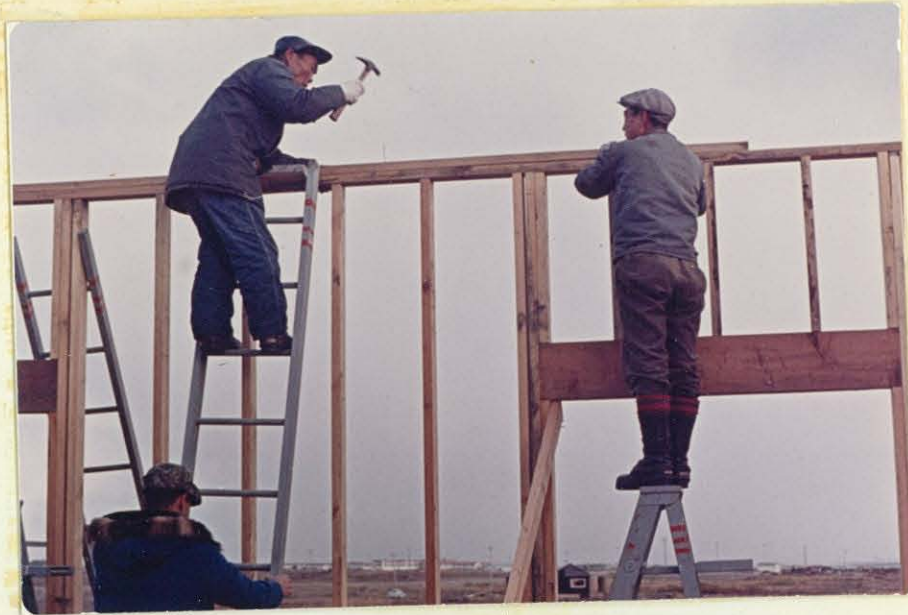
Wassili Berlin with hammer, Paul Tinker living dangerously, and Jim Geerdt holding ladder while working on an addition to the Service Building. Photo by J. L. Hout, 9-30-65.
