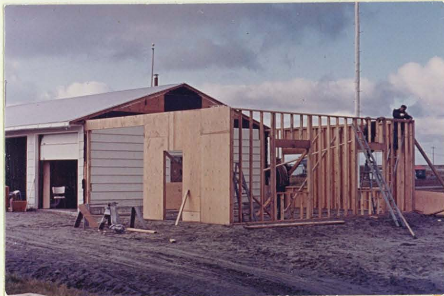
This addition will provide space for a heated workshop. The level fill to the right has been surfaced with gravel and will be used as a parking and equipment storage area. Photo by J. L. Hout, 9-30-65.
