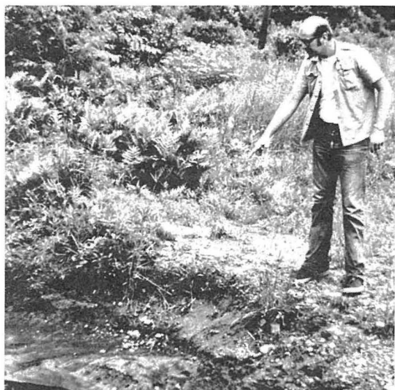
FIG. 14.1.3. Severe sheet and rill erosion at access road where culvert was installed on bank of stream crossing ROW.
