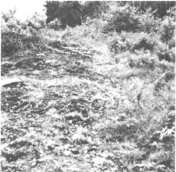
FIG. 21.1.3. Equipment cut exhibiting severe sheet and rill erosion on the ROW, in the spring, 1975 (Photo Station 7).
