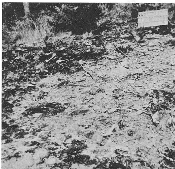
FIG. 20.1.3. Slight sheet erosion on ROW, in summer of 1975 (Photo Station 6).
