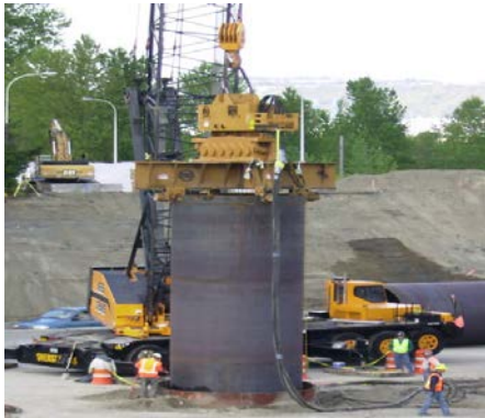
Figure 5: A vibratory hammer sets a piling for a bridge in a process very similar to driving pipe for mooring dolphins (WSDOT 2008).
