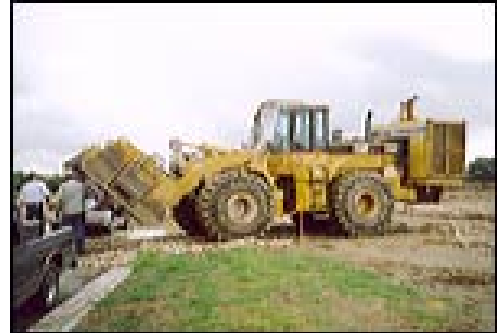
Figure 3: A Series II Profiler Roto Trimmers similar to those used to remove organic overburden (Joe Bland Construction, L.P. 2006)
