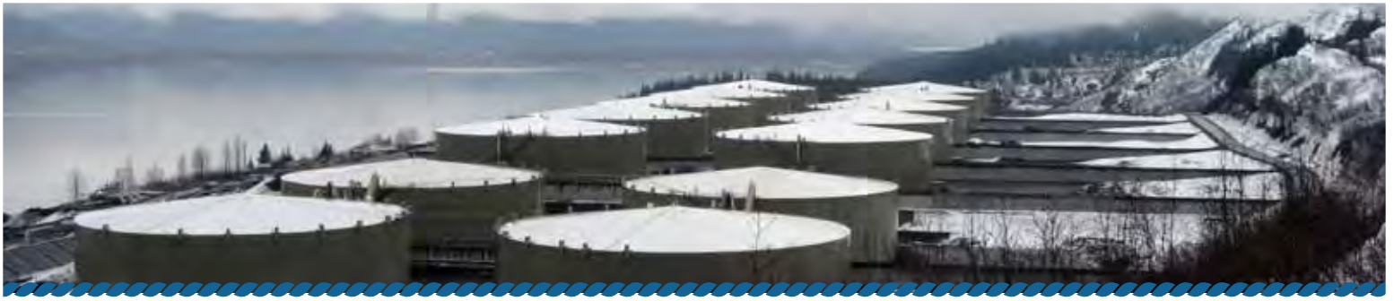
↳ These tanks at Alyeska's Valdez terminal store oil that comes in from the trans-Alaska pipeline until it can be loaded onto tankers for shipment south. Photo by Stan Jones.
