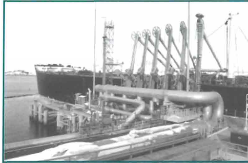
New equipment at Berths 4 and 5 collects oil vapors from tankers during crude oil loading. Photo by David Predeger.
