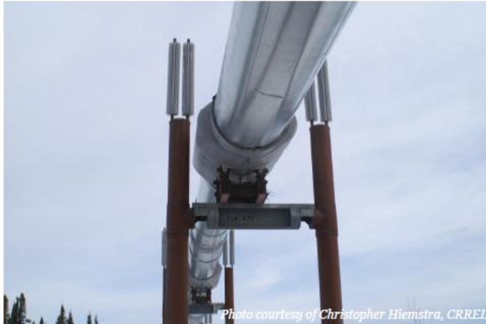
Figure 30. TAPS Aboveground Pipeline with Thermosyphons
