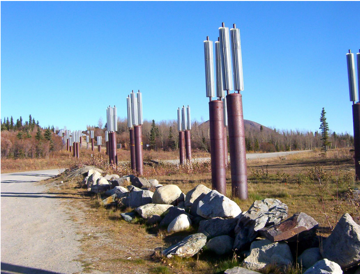
Figure 29. TAPS Buried Segment with Thermosyphons
