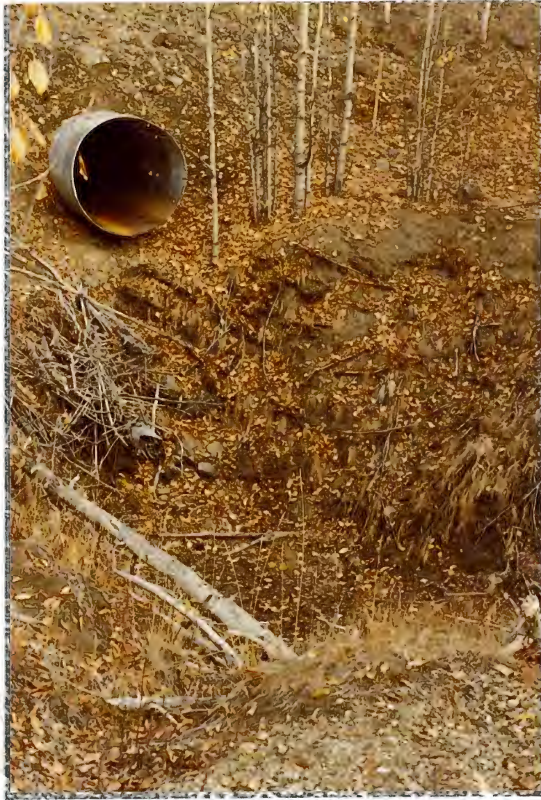
9/16/81 - Unnamed Creek (RX 128-1) looking upstream to Alaska highway CMP outlet and scour hole.
