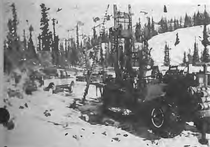
Geotechnical crew sets up drill to take core sample along the Alaska Highway near Marsh Lake in Yukon.
