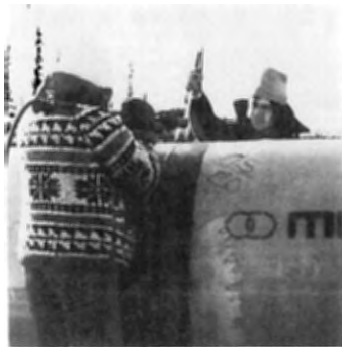
Labourers apply heat to completed weld at Quill Creek test facility, northwest of Whitehorse.
