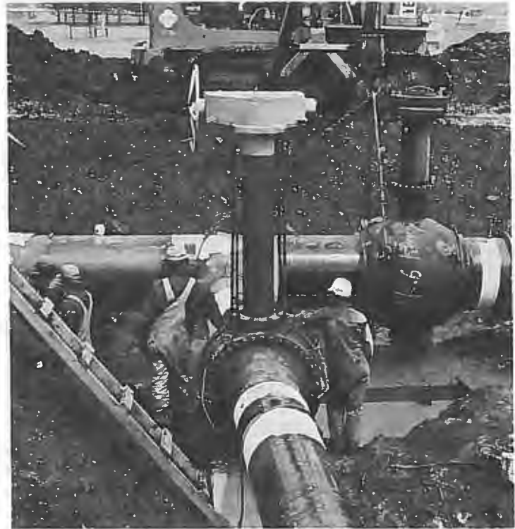
Final tie-in to the ANG system in the Crowsnest Pass area of South B.C.
