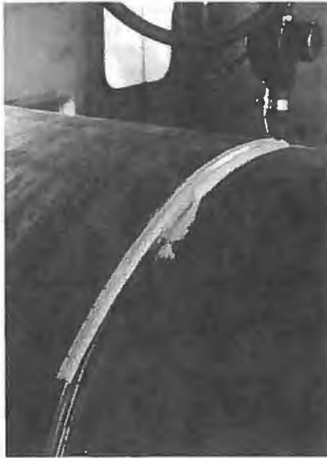
1,067 mm (48 in.) pipe for compressor stations is "prefab" welded using submerged arc method.
