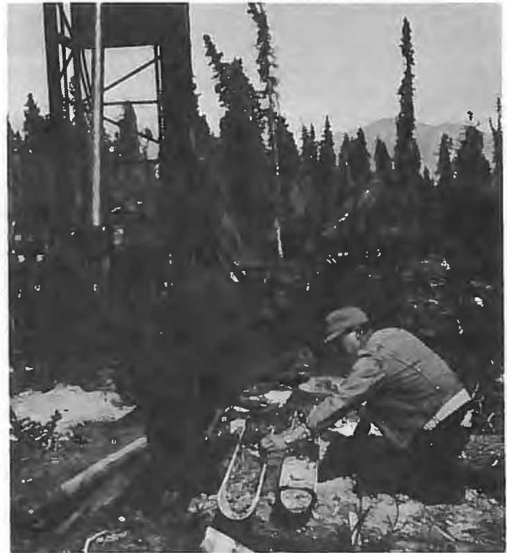
A hydraulically-powered sonic drill obtains samples from coarse soils at a compressor station site near Destruction Bay.
