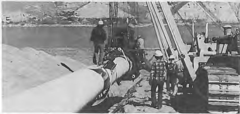
Pipe is wrapped with protective plastic tape and lowered in to the ditch on the west bank of the South Saskatchewan River in Alberta.
