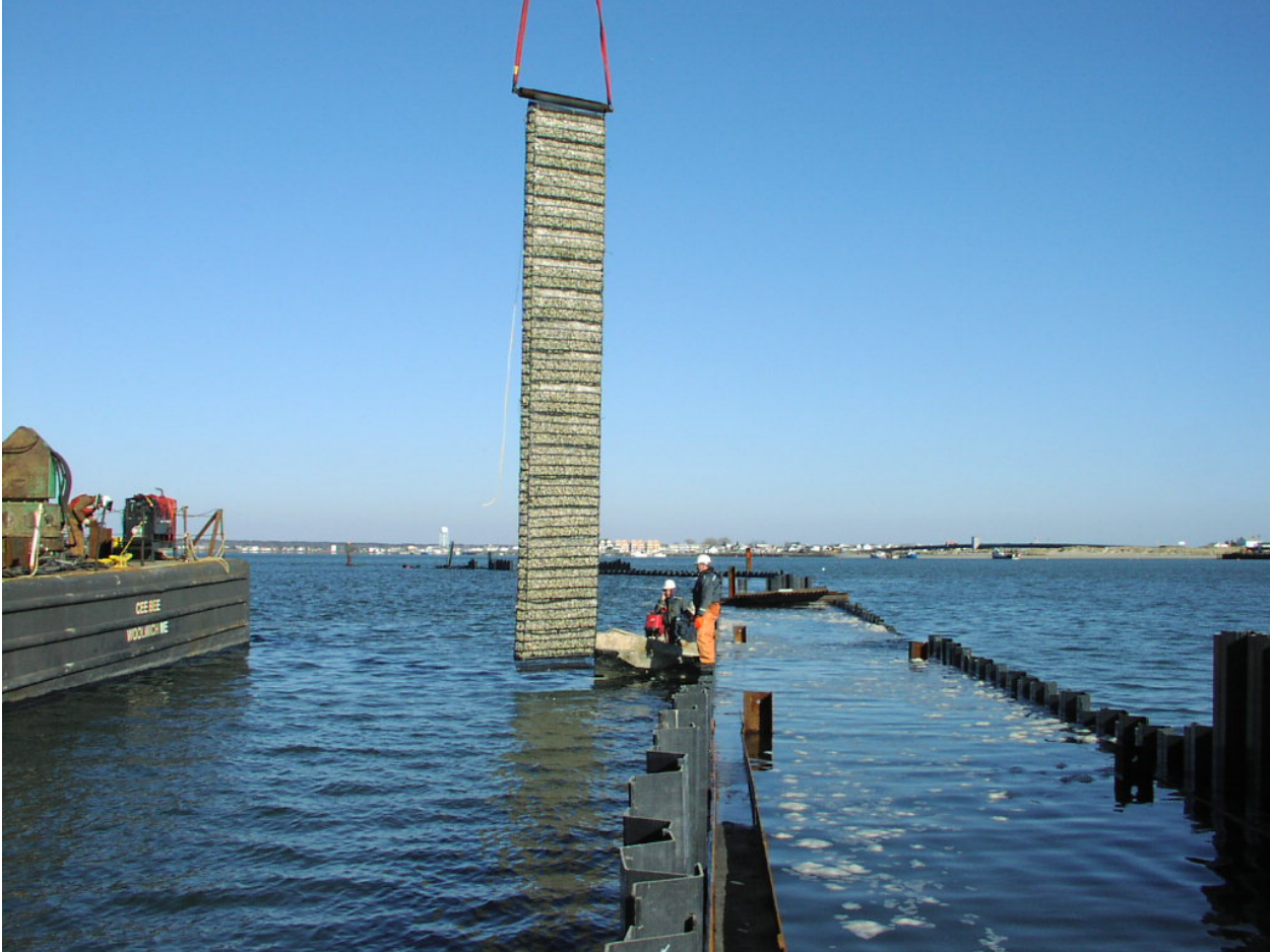
Figure 12. Mattress placement at Seabrook, NH, Section 227 project (photograph by Scott Leonard, New England District)
