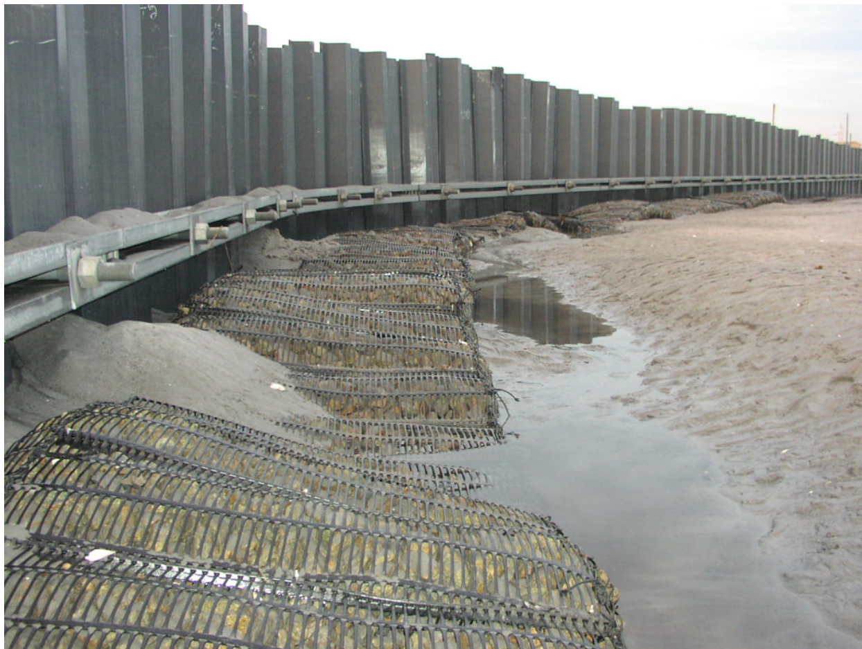
Figure 13. Scour apron at Seabrook Section 227 project at low tide (photograph by Scott Leonard, New England District)
