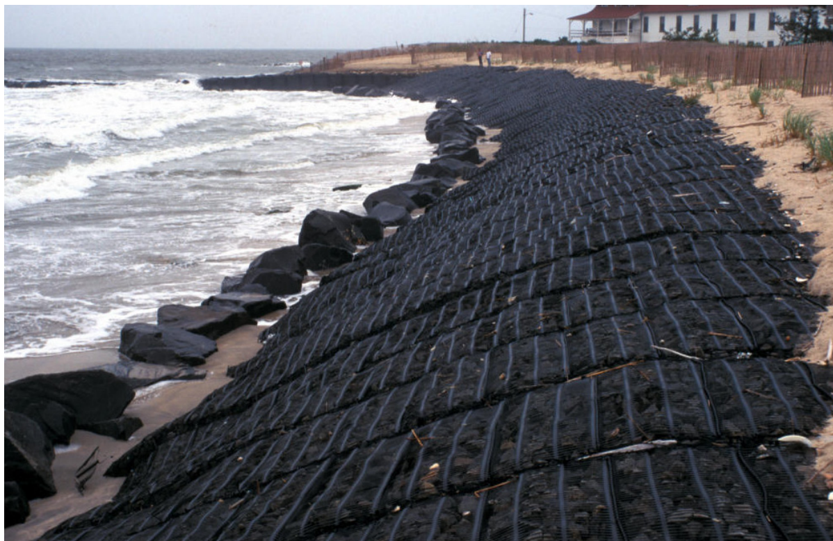
Figure 7. Cape May State Park shore protection mattress revetment shortly after placement (photograph from Jeffrey Gebert, Philadelphia District)
