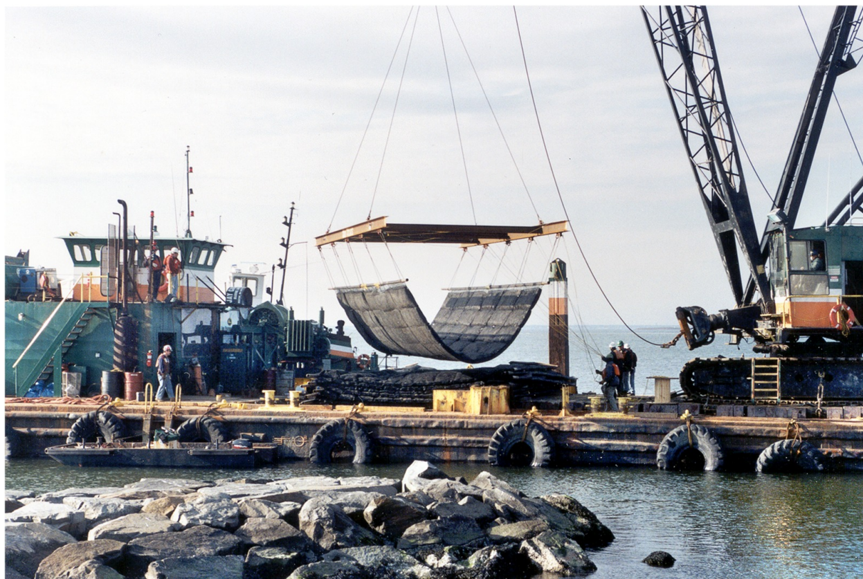
Figure 9. Barnegat Lighthouse with mattress placement underway (photograph provided by Jeffrey Gebert, Philadelphia District)
