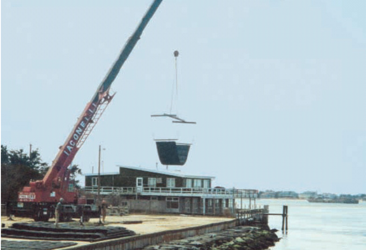
Figure 3. Installation of mattress at Barnegat Inlet, NJ (photograph courtesy of Tensar Earth Technologies)
