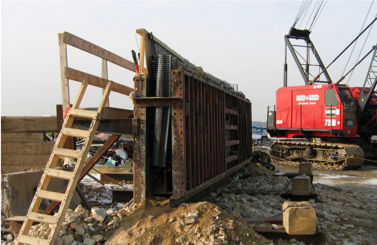
Figure 6. Construction jig used to fill marine mattresses at Section 227 project in Seabrook, NH (photograph by Kevin Knuuti, CHL)
