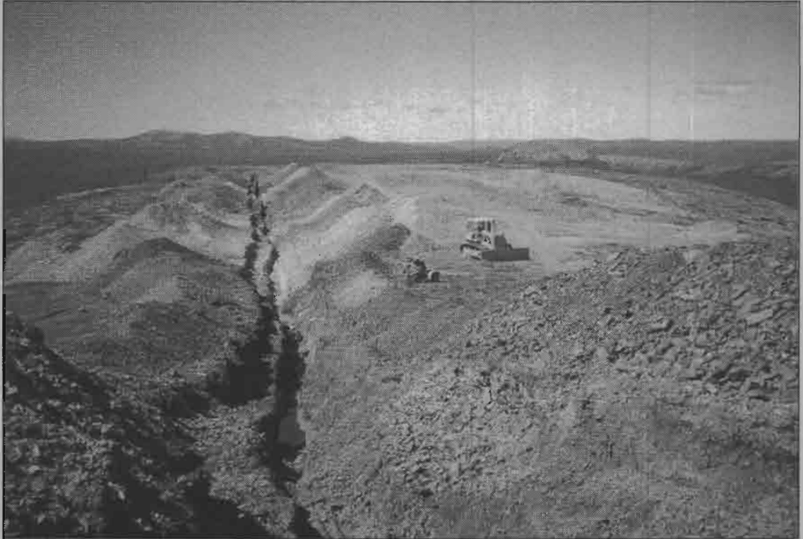
Excavator and bulldozer trench on Lewis Ridge, Donlin Creek property, southwestern Alaska. Trench is approximately 1,300 feet long and part of a 3.7-mile trenching program by Placer Dome Exploration Incorporated during the 1997 and 1998 field seasons. Light-colored rock is igneous dikes and sills, and darker rocks are Kuskokwim Group shale and graywacke.
