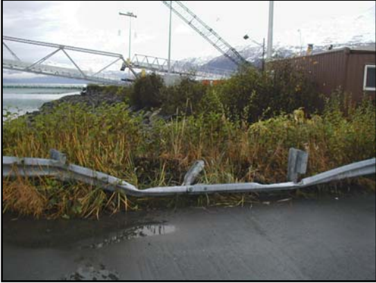
Damaged Railing at East Approach Ramp
