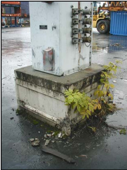
Damaged Power Pedestal
