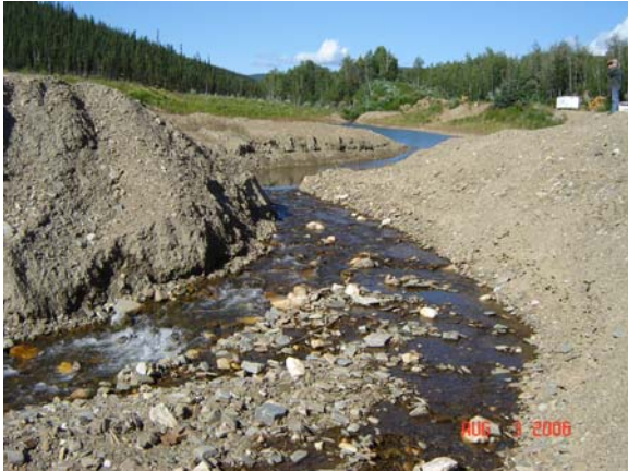
Photograph 4. View of the constructed outlet channel between Ponds 1 and 2, looking upstream into Pond 1, August 2006.
